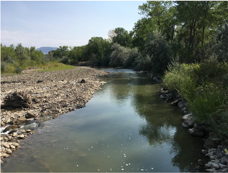
Figure 2.6.1.3. Short Ditch Boulder Weir Diversion
