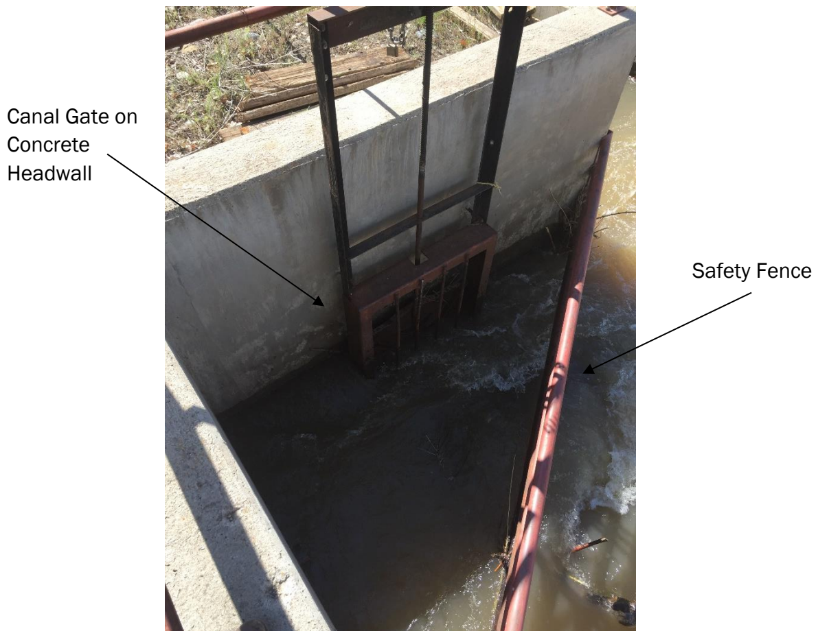
Figure 2.8.1.4. Canal Headgate with Safety Fence
