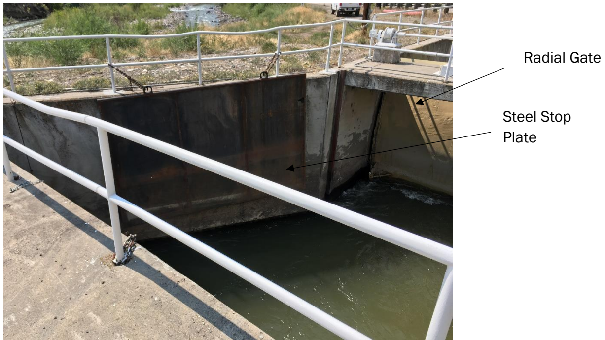
Figure 2.2.1.5. Radial Gate and Steel Stop Plate within Fire Mountain Canal Intake Structure
